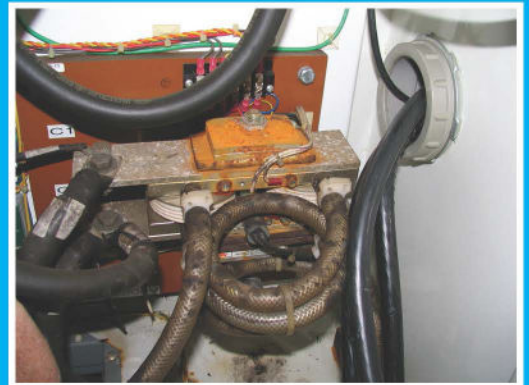
SCR contactor rusty from condensation
