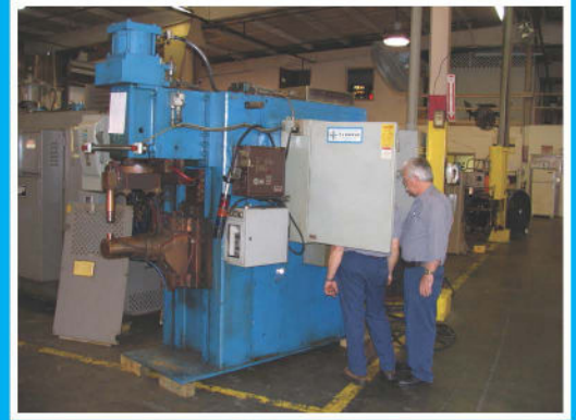
Surveying the damage to the contactor cabinet
